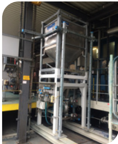
Container- emptying station with DASAG –Powder Pump
