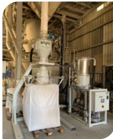
Spillage return system of a packing system with bag emptying station and BIG BAG filling station
