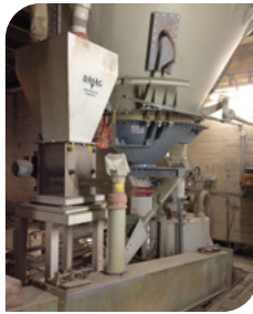
Bypass dust dosing system
