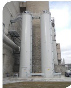
Silo -system for iron(II) sulphate
